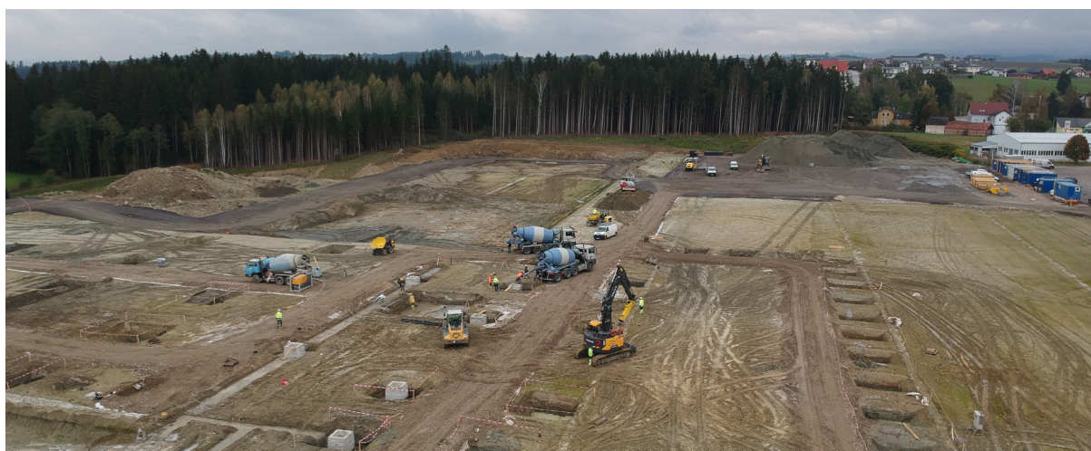
A large construction site where the fast installation of the TRM Piling Systems was fully used.
