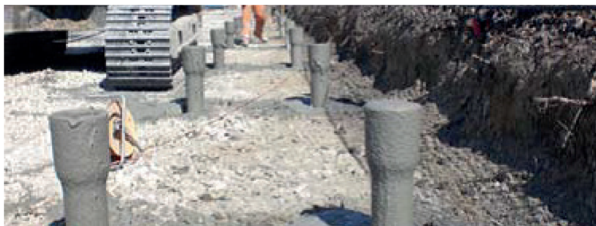
The pile grids with 3.0 metre distance consist of two grouted ductile iron piles which can be alternately loaded by wind loads in compression and tension.
